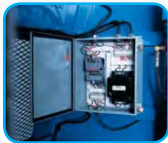
BE-TS Control Panel
