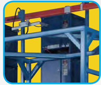
BE-TS Buss Duct
